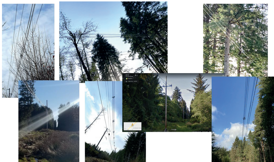
Figure 5: PacifiCorp Covered Conductor Effectiveness Examples
