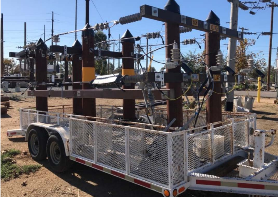
Figure 1: Covered Conductor Mobile Trailer
