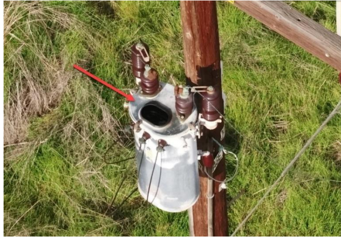
1 2 Figure JK- 5: P572459, 4/9/2020, Transformer 3 lid missing.
