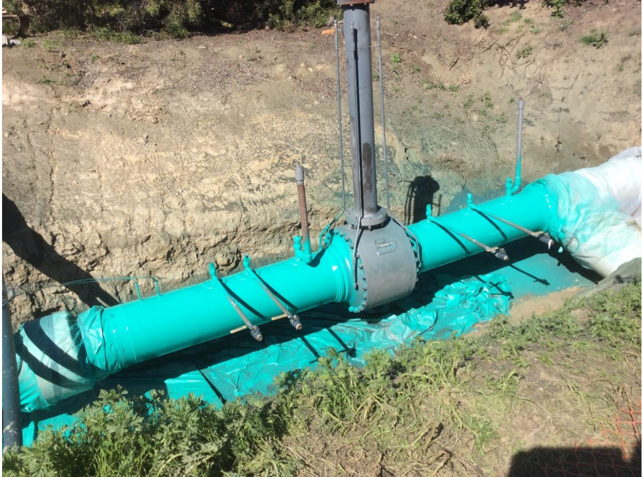
Figure 3: Mainline Valve Assembly With Instrument Piping
