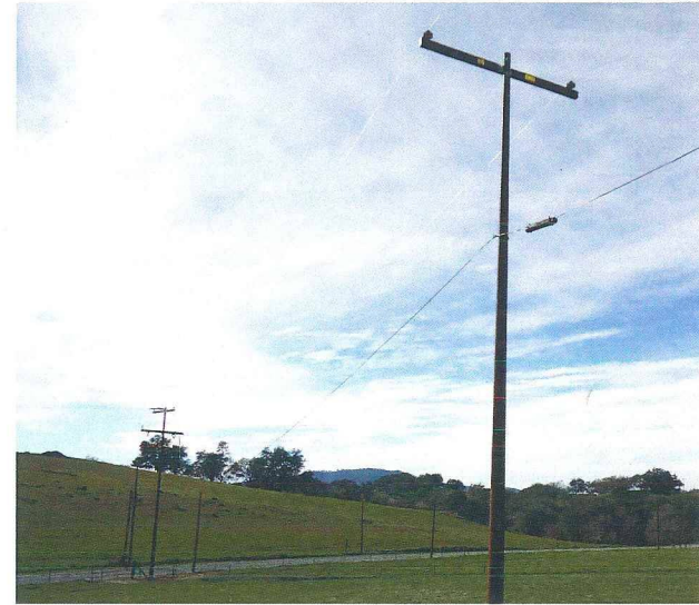
The new steel poles replacing the existing ones have a reddish-brown appearance similar to wood and are known as "weathered steel" poles.
