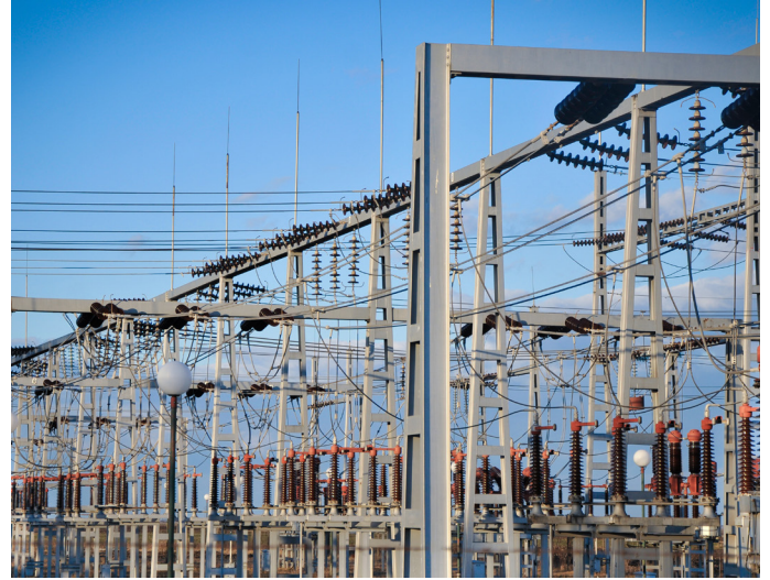
An above-grade transmission substation infrastructure.
