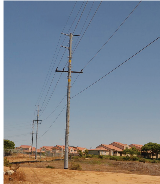
Steel poles, like the one pictured here, will replace wooden poles in an area of Otay Mesa starting sometime after February 2019.
