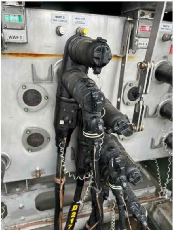
FIGURE 2 PHOTO 2-FRONT VIEW EQUIPMENT ELBOW 15KV R-800 DOUBLE INTERFACE
