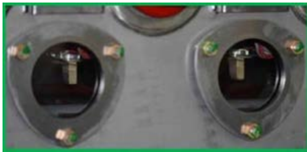
VISIBLE OPEN SHAFT "OPEN"
