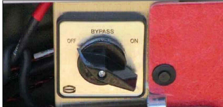
FIGURE 5 BYPASS SWITCH (E)
