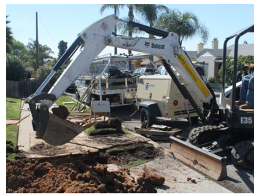
Trenching in both public streets and private property is a necessary part of the undergrounding process.
