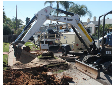
Trenching in both public streets and private property is a necessary part of the undergrounding process.
