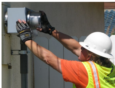
Crews will need to access meter service panels so they are ready for new underground service.
