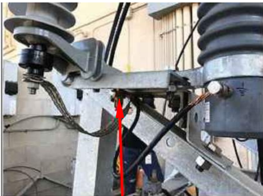
GROUND CONNECTION POINT ON FRAME FOR SENSORS AND ARRESTORS
