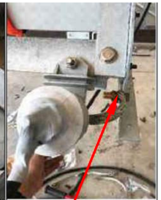
LOAD-SIDE ARRESTOR GROUND
