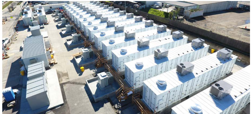
Escondido Battery Energy Storage System project
