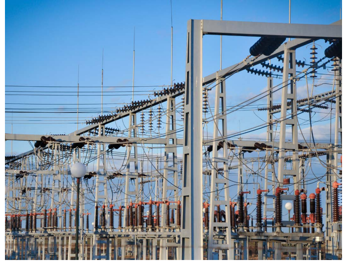
An above-grade transmission substation infrastructure.
