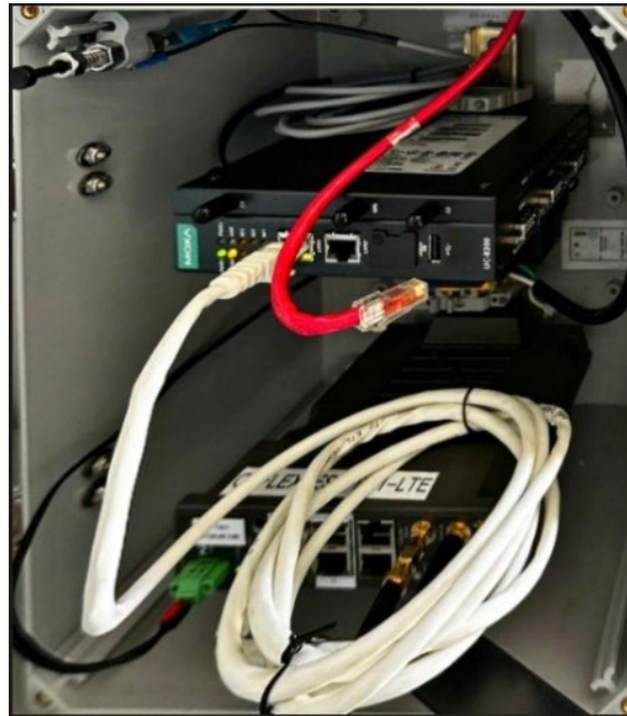
Figure 4-9. Modbus Gateway Disconnection from MBESS Local Controller to Emulate the Communication Loss Scenario
