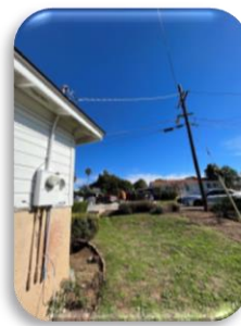
Source (pole or midspan attachment) serving meter - taken from meter panel location towards source
