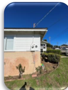
Panel location showing at least 5' of space to the left and right of meter location, from ground level to the roof & point of attachment, and working space in front of meter location
