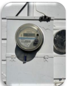
Close up image of meter to identify meter number
