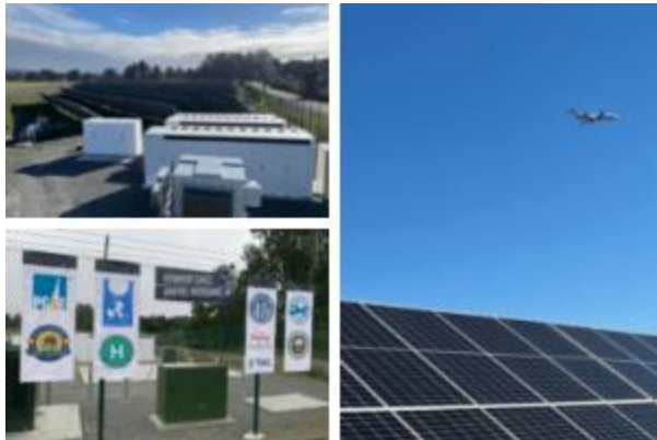
Redwood Coast Airport Microgrid (RCAM)
