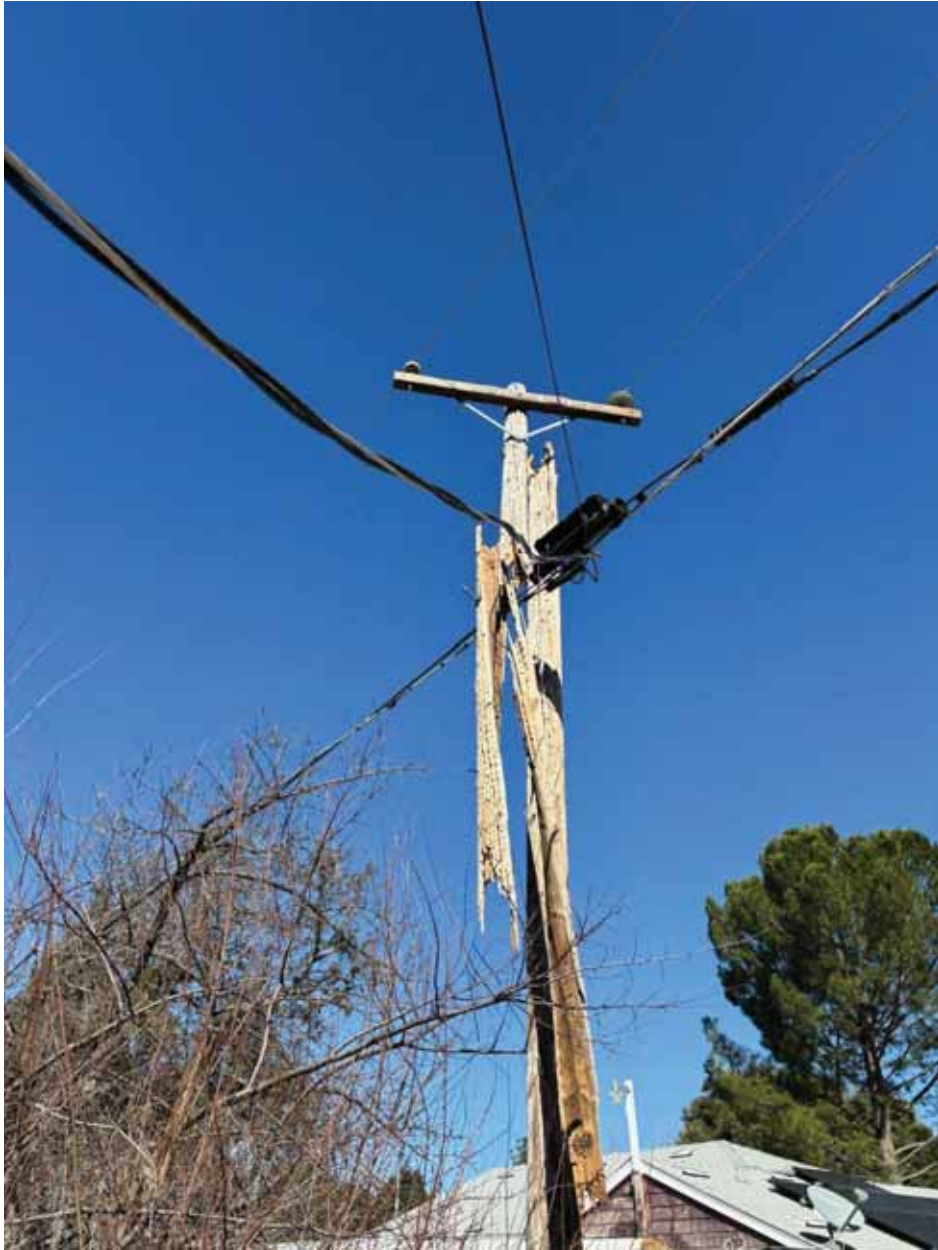
Figure 23 - Item #1 P42621J Broken Pole
