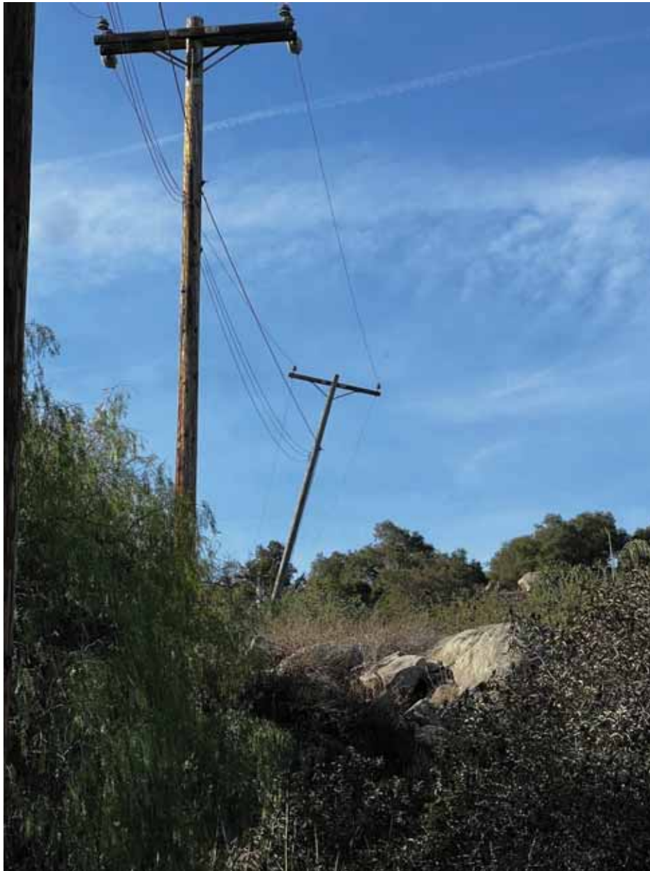
Figure 25 - Item #3 P133349 Broken Pole
