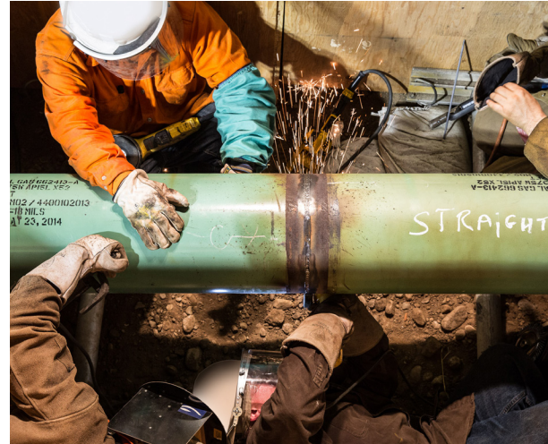
SDG&E has upgraded more than 35 miles of transmission pipeline in San Diego County as part of our Pipeline Safety Enhancement Plan.
